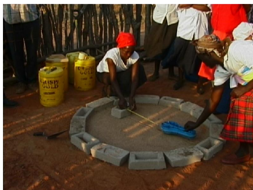
Fig 14: Sanitation in Tsholtosho (2001) Women build latrines themselves having made Interlocking cement blocks used to line the pit
