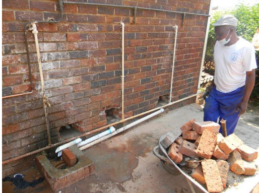
Hatcliffe waste water reticulation for showers
