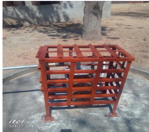
Submersible pump installed and secured at Imbizo Pry
