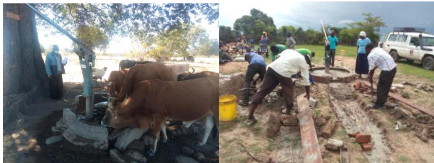
Fig 1 The quest for Headworks- livestock watering from a broken apron at Mutswakatira water point and headworks construction at Fiomumwe Water point ward 10 Gutu
